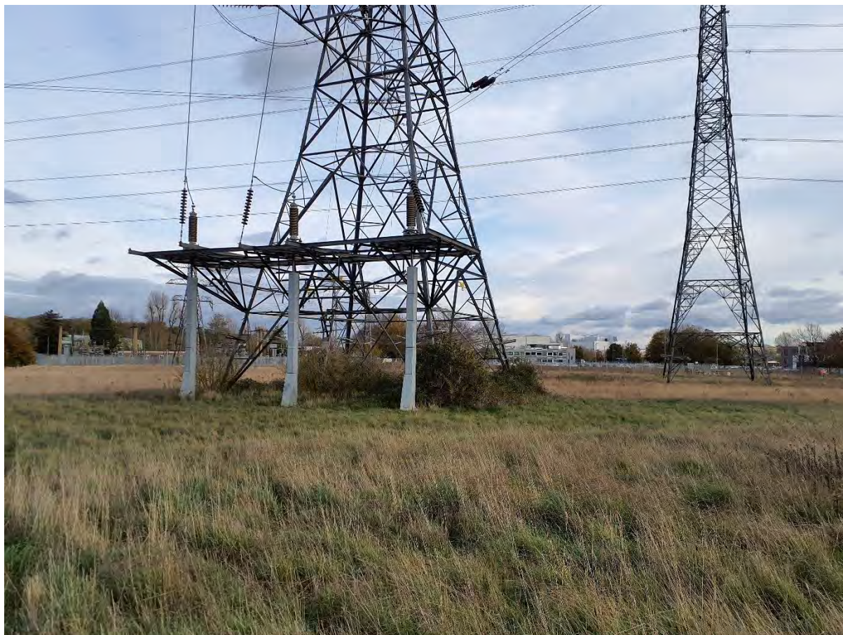
Figure 12 – Pylons at the southwest of the site.
